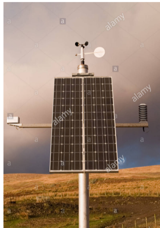
(b) Meteo station (solar)
